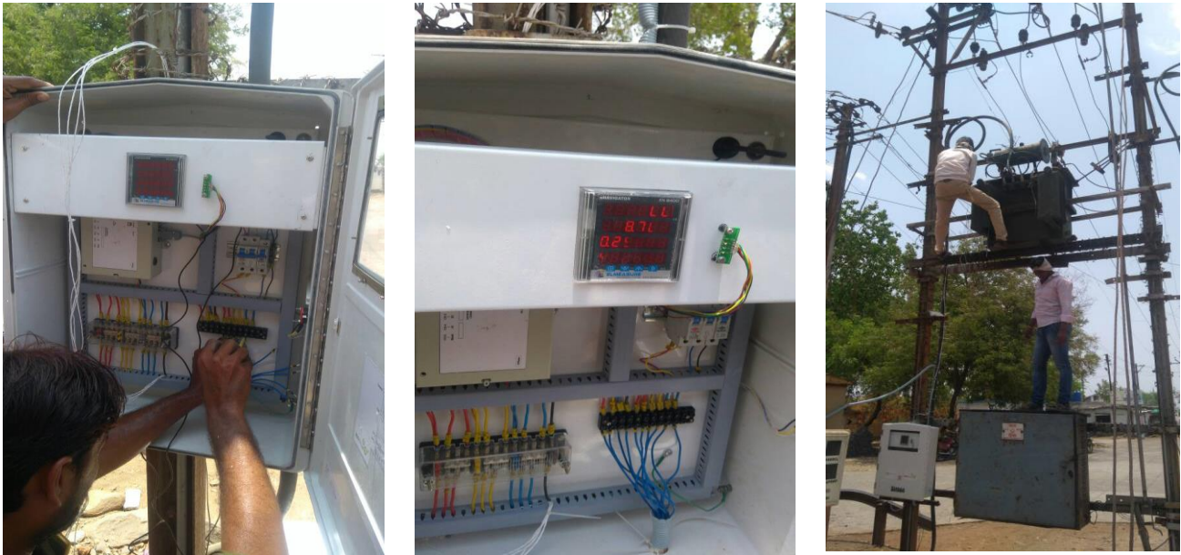
Figure 1. Transformer Monitoring unit
